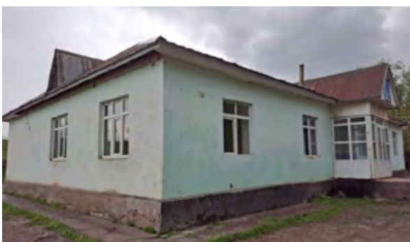
General education secondary school of №16, Town Langari Shoh, Village Kuli Kalon, Tojikobod District, damaged in the earthquake on April 13, 2025
